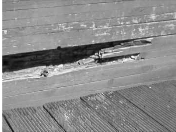
Figure 4: Damage in the beam
