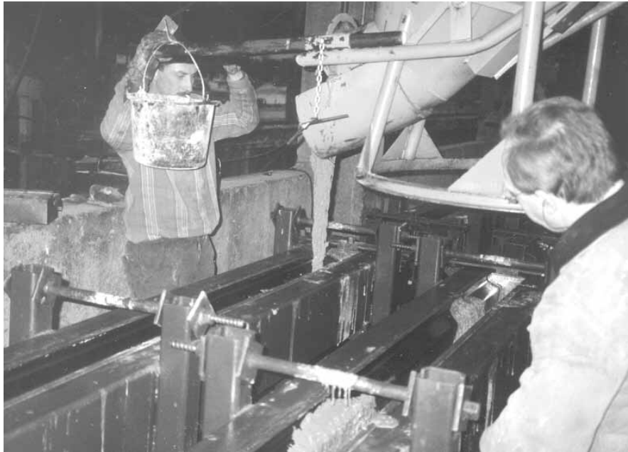
Fig. 3. Casting a UHPFC beam by Hurks Beton, the Netherlands, for the viaduct Bourg-les-Valence (France).
